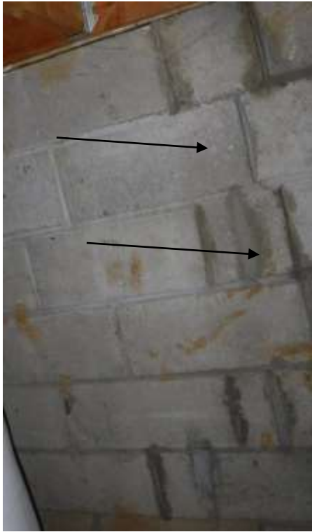
Figure 6 Example of cracks on foundation; see structure comments pg.2. There was perimeter storage and clutter in garage; limited view.
