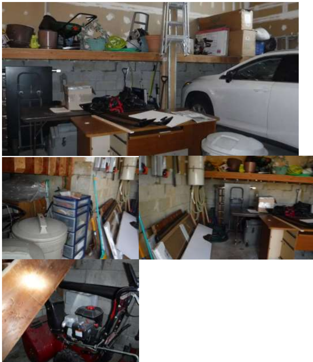
Figure 5 Inaccessible outlets, perimeter, flooring; car, storage, clutter in garage. Inspect all areas and outlets when storage removed. Water/moisture/efflorescence stains on foundation.
