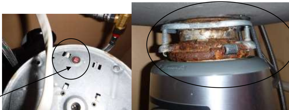
Figure 7 On left, red reset button if tripped, rest to restore power. The right photo is the corrosion on drain basket and garbage disposer connector; have licensed plumber evaluate for replacement.
