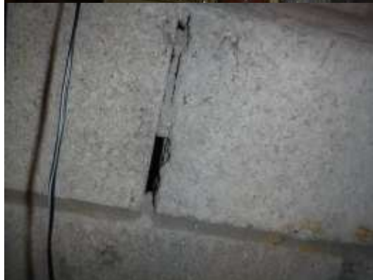
Figure 9 Example of missing mortar; have a structural mason evaluate all cracks, missing mortar when clutter removed.
