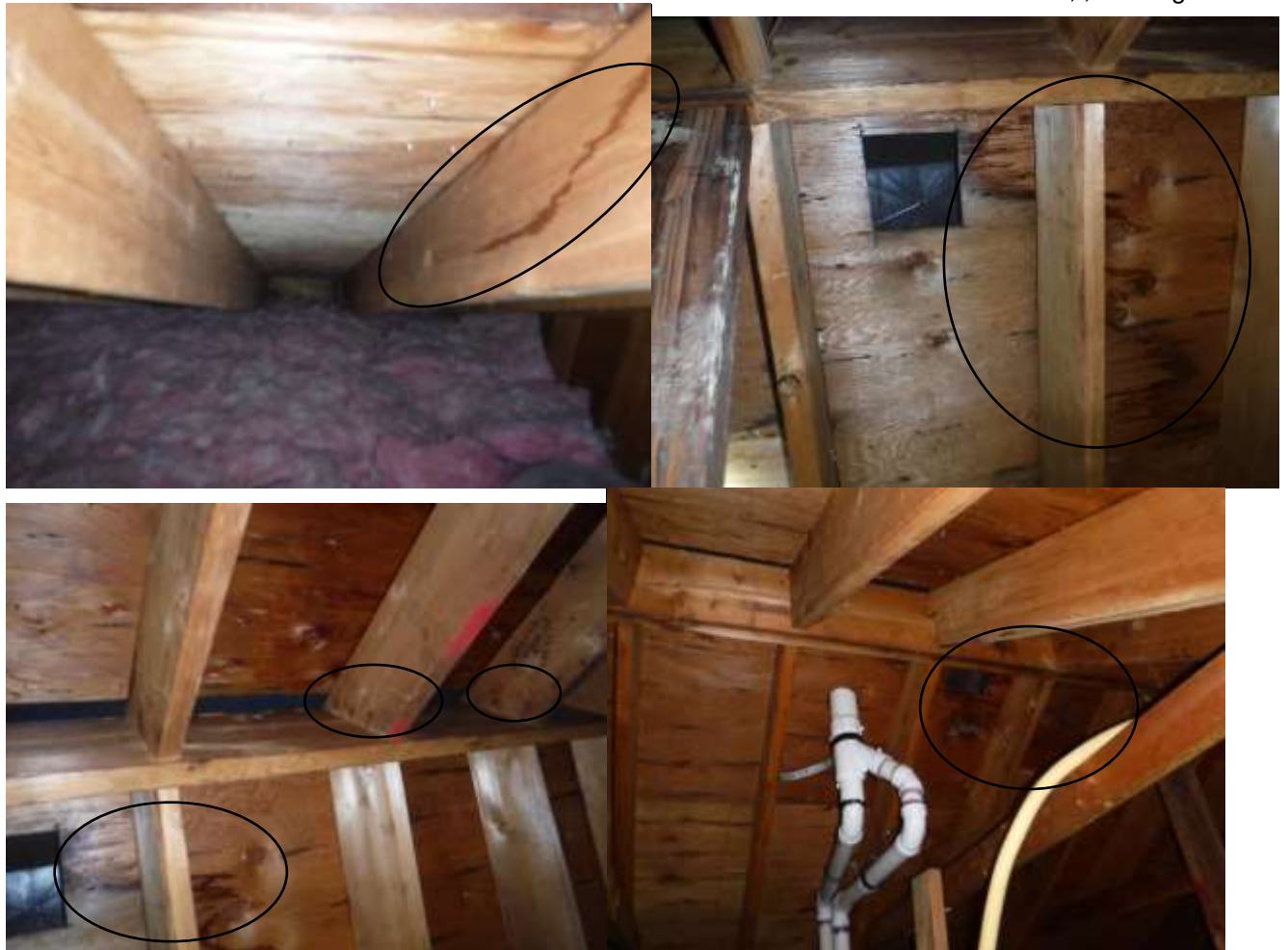
Figure 2 Examples of water stains (camera zoom); inaccessible. Follow up with roofer to make sure water stains in attic are old and not active. Recommend a secure catwalk in attic for roof inspection and for servicing the HVAC equipment, ducts, etc.
