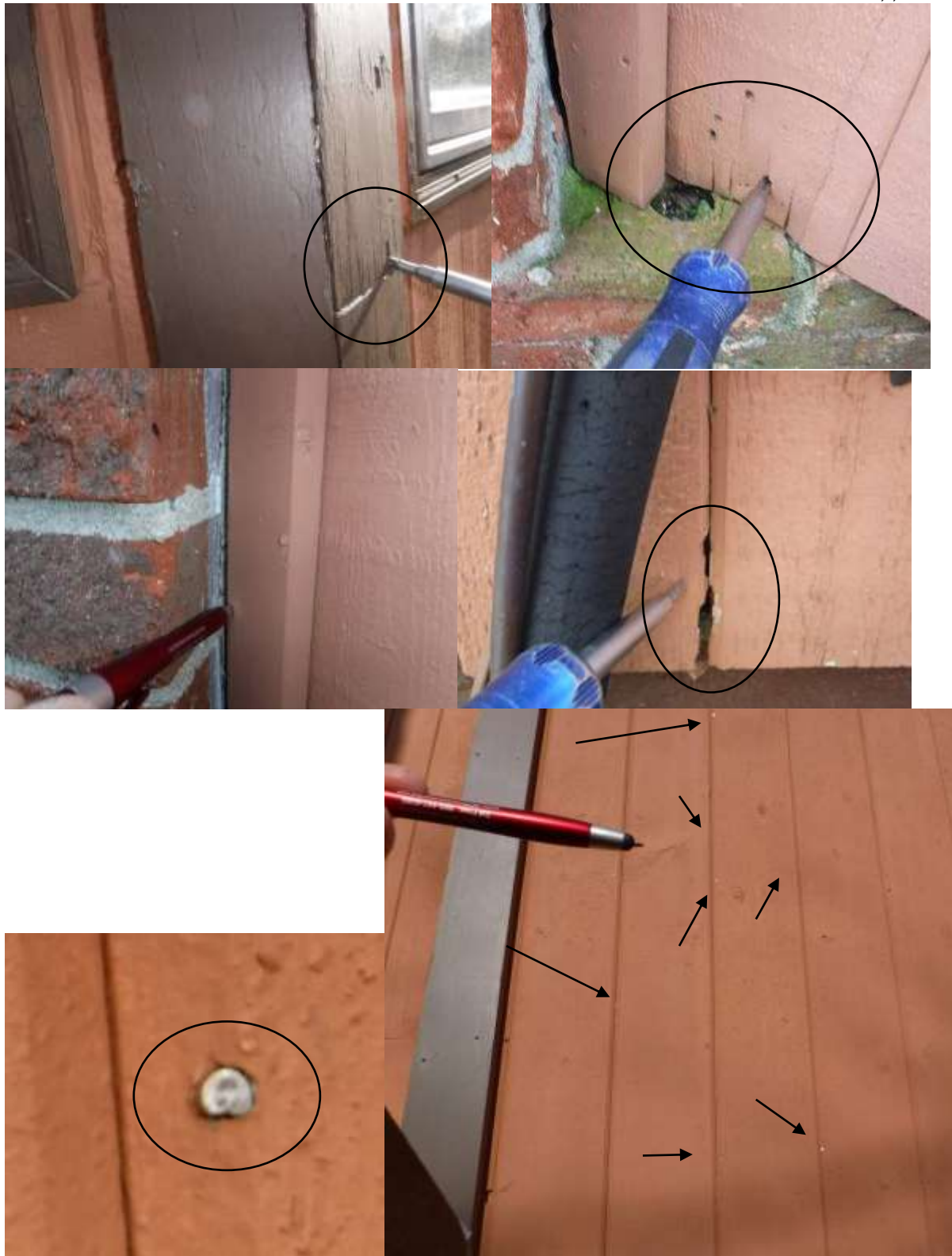
Figure 3 Numerous shiny nail heads on siding, wood siding & trim rot/water damage; further evaluate with siding contractor.
