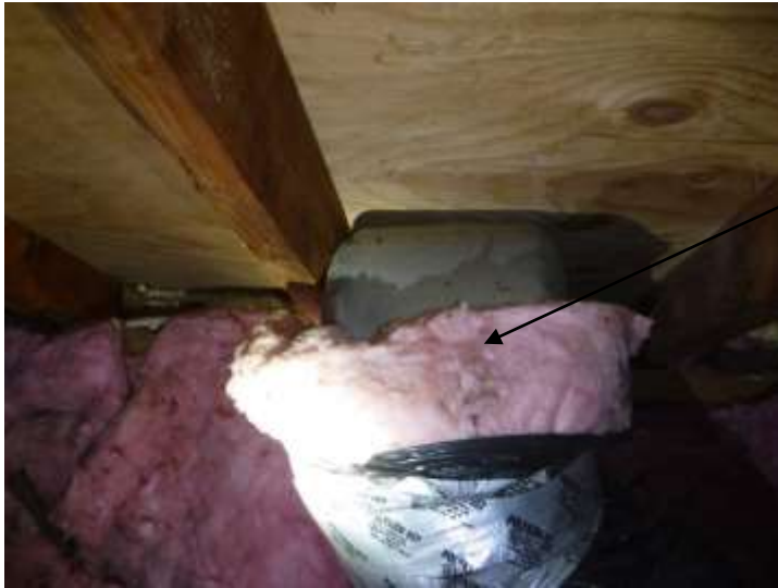
Figure 10 Example of loose ducts ; recommend adding HVAC strapping/ties where needed in the attic/basement/home.
