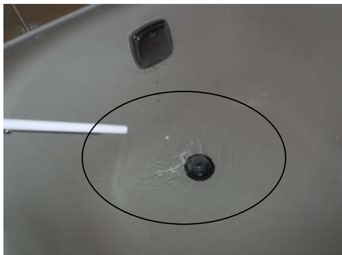
Figure 8 Slow drainage; have a plumber evaluate drainage and advise on repairs.
